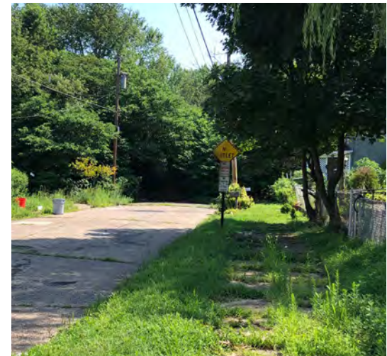
Sidewalks and curbs in need of replacement
