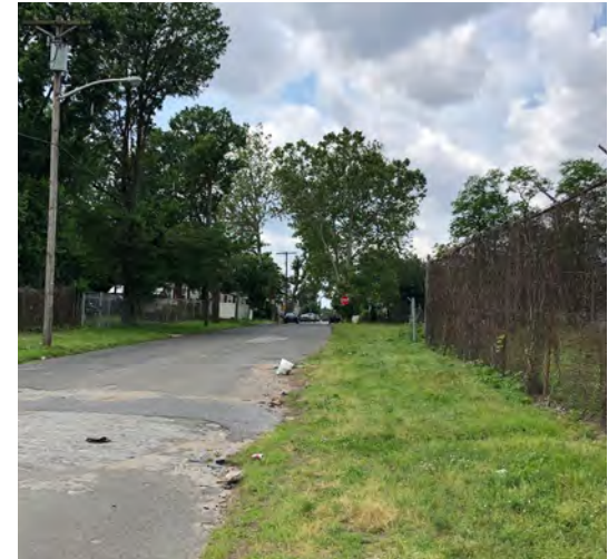
Missing sidewalks and curbs
