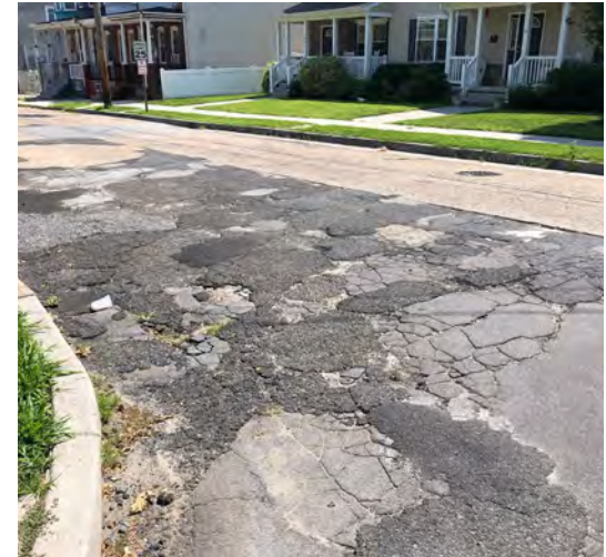
Typical street identified as in poor conditions
