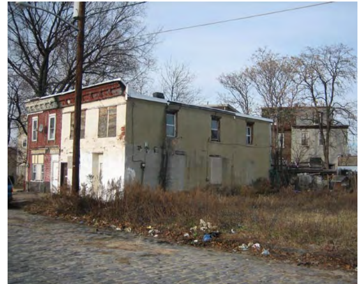
Deteriorated street conditions on State Street, top, and lack of sidewalks on Main Street.
