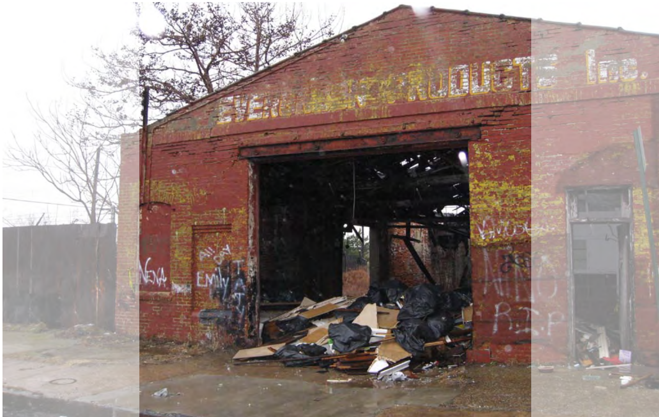
The Evergreen site near Front and Erie is a small, known contaminated site that is the source of much concern in the neighborhood. Source: SOW
