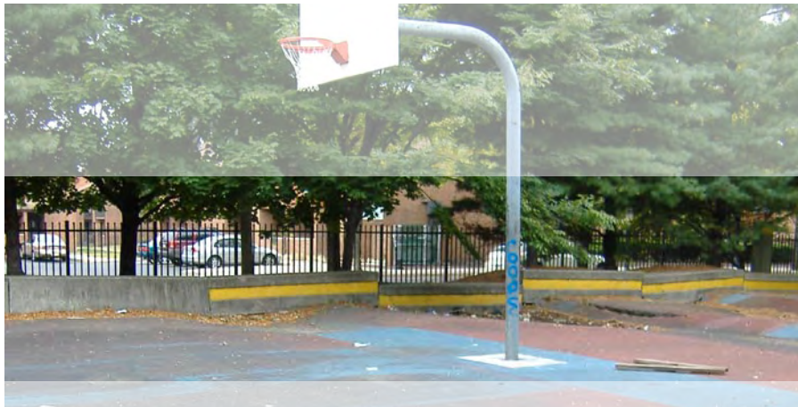
Ground settling at Northgate Park necessitates major park rehabilitation.
