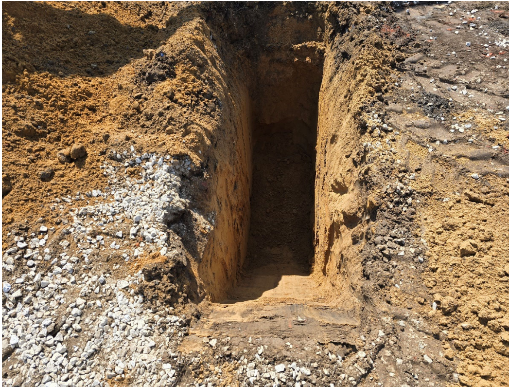
September 12, 2024 – Test pit TP-11
