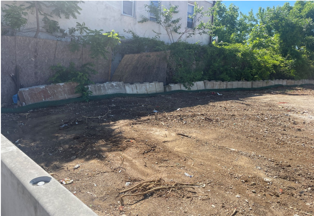
June 7, 2024 – Photo taken by Montrose of former stained soil area (AOC-9b) following post-excavation and backfill at Block 331.
