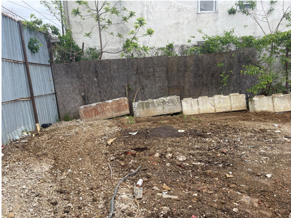
May 13, 2024 – Photo taken by Montrose of stained soil (AOC-9b) at Block 33 prior to excavation.
