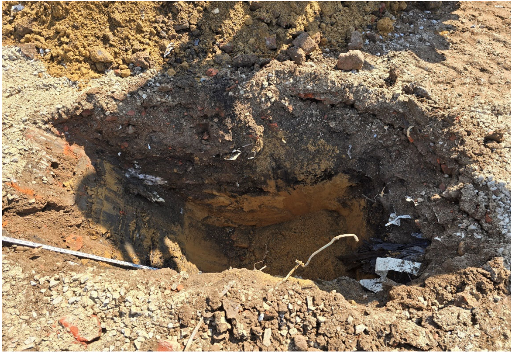
September 12, 2024 – Test pit TP-6
