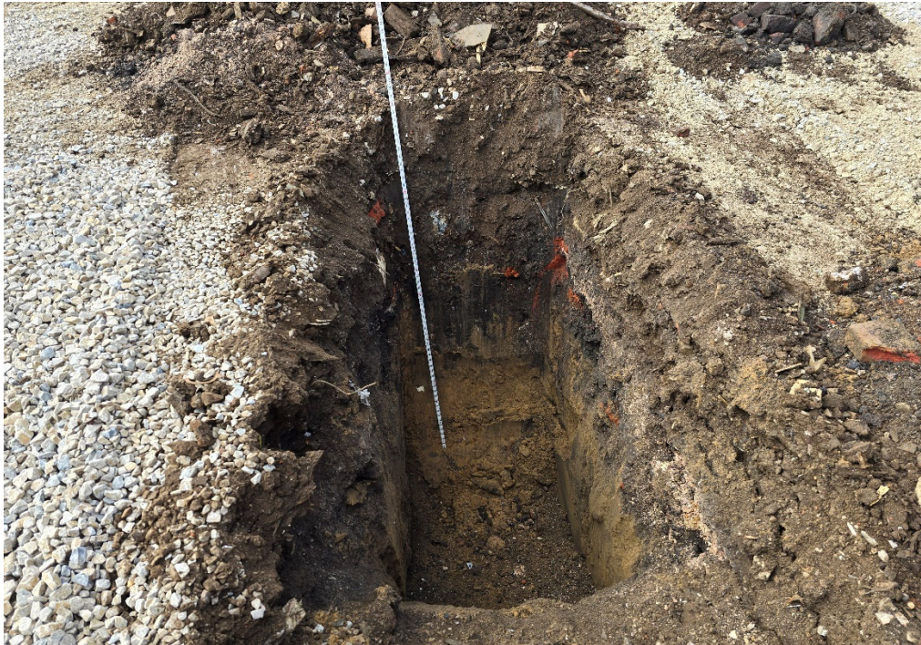
September 12, 2024 – Test pit TP-3
