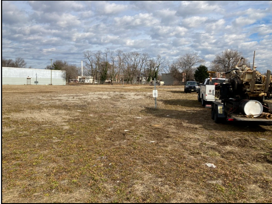
Additional AOC 9-1 delineation samples installed in the southeastern portion of the site
