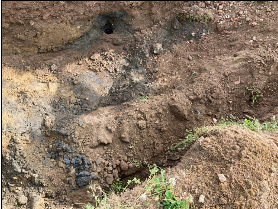
Stained soils in the vicinity of the fill port of AOC D
