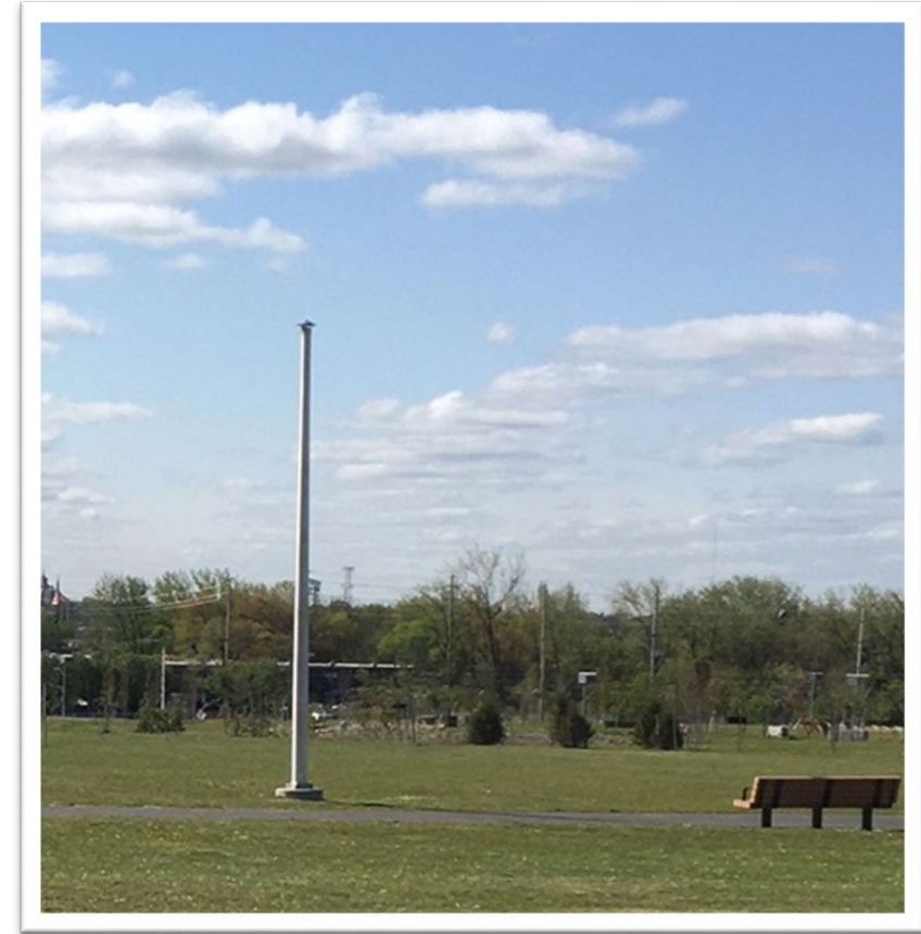
Vent from Passive Gas System Credit: Jennifer Taylor, BRS, Inc.
